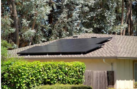
Non compliant street-side roofs with exposed and metallic mounting hardware and lack of symmetry in application of equipment
