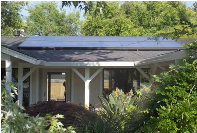
Street-side application with metallic look and exposed mounting hardware
