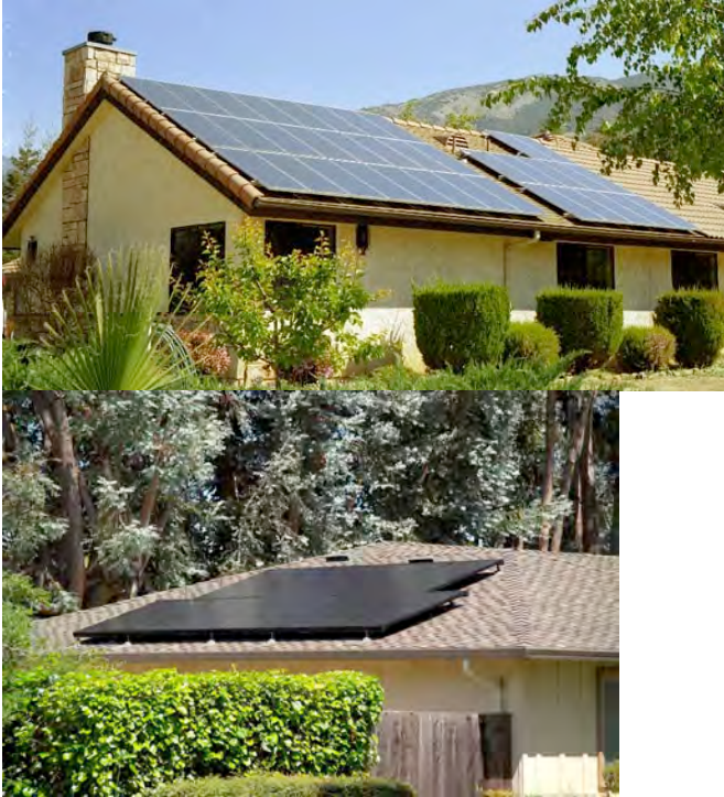
Non compliant street-side roofs with exposed and metallic mounting hardware and lack of symmetry in application of equipment
